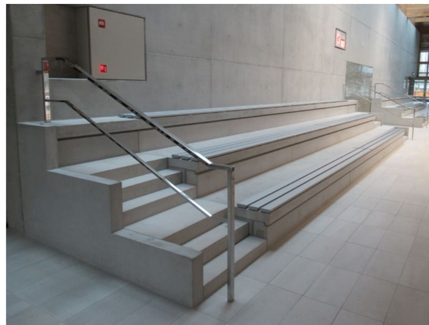
A9 Prefab betonnen tribune-elementen met houten zitplank.
